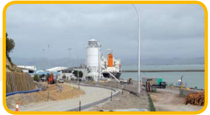
Right on track...the new road in the Hirini Street Project sweeps around the side of Kaiti Hill.
