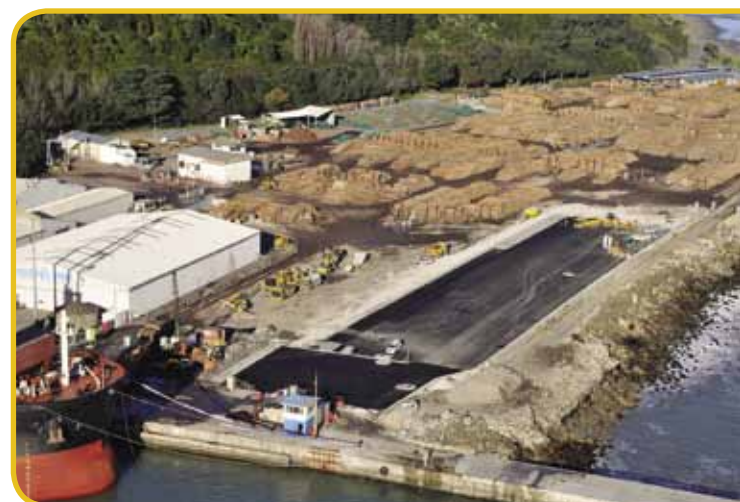
A bird's-eye view of the first stage of the multi-million dollar asphalt project underway at Eastland Port.
